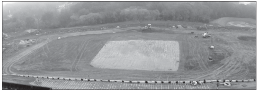
A composite of two photos taken from the Classic Center Foundry Street Parking Deck showing the work area for the Multimodal Transportation Center. Off to the right is East Broad Street.
